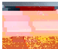
Fire alarm call point
